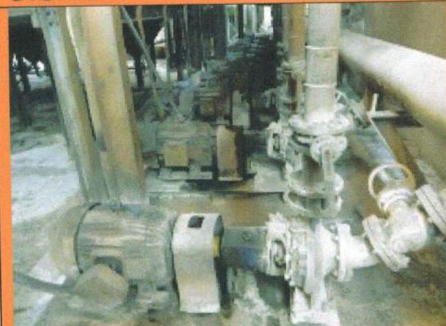
48. Bomba centrífuga Meganorm KSB
